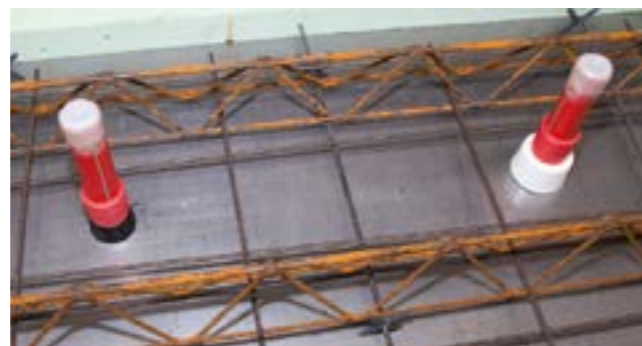
1. Type of connection: visible sprinkler
