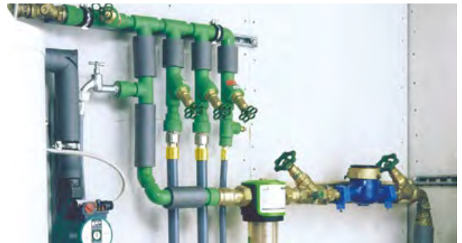
House connection station
