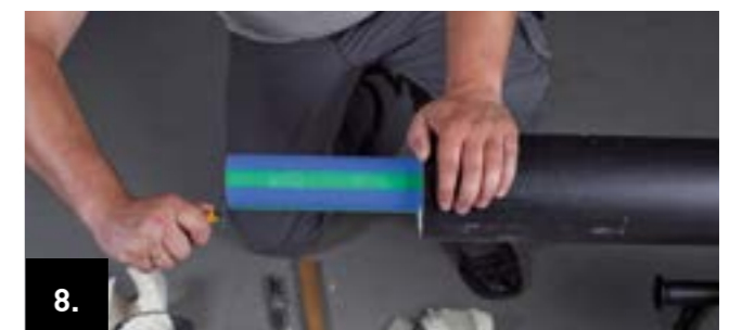
8. Clean the stripped carrier pipe and deburr the pipe end both internally and externally.
