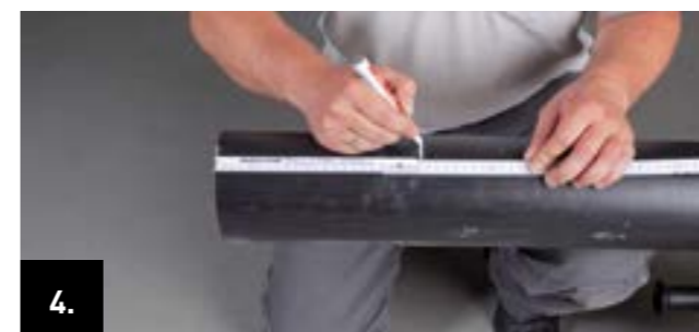
4. Mark the stripping length of 22.5 cm from the pipe end on the casing pipe.
