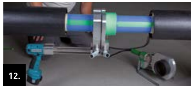
12. Align the welded joint with the pulling device and fix for a short time. Further processing takes place after the specified cooling time has elapsed.
